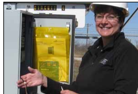
Danelle Taylor runs fiber-optic cables at the Osceola substation to the communications shelter to enable remote control of some system switches.
